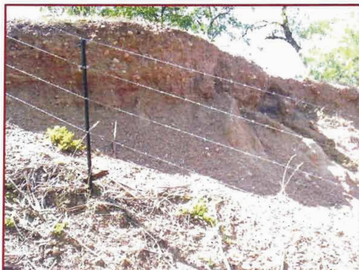
Photo 9 – Erosion scarring along the gully banks
